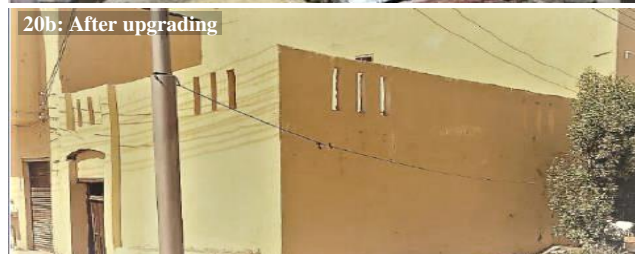
Fig. 20a and 20b. Unfinished walls were plastered and painted, and missing parapets were built (Photo credit: Authors)
