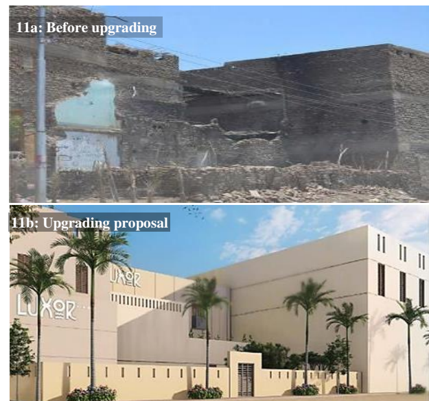
Fig. 11a and b. A proposal to upgrade the visual character of decayed façades by completing, straightening, plastering and painting of unfinished walls. (Authors)
