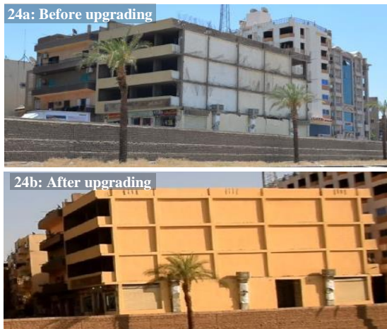
Fig. 24a and 24b. Finishing of the remaining parts of partially demolished buildings (Authors)
